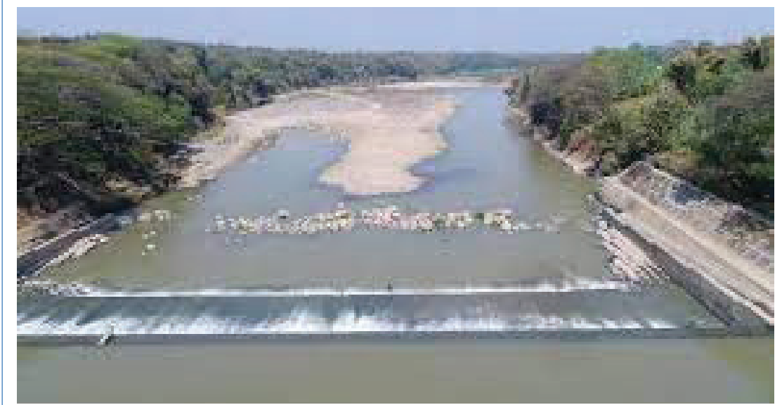
Photo 3-24: Typical damaged ground sill
