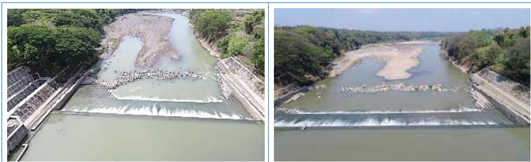
Photo 3-25: Example of progressive groundsill damage based on field observations
